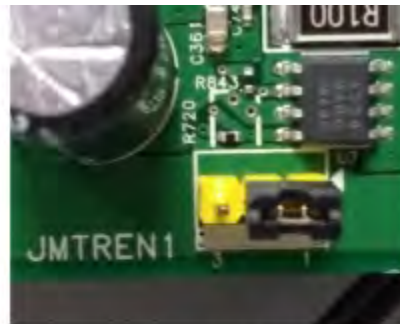
Interlock bypass enabled
