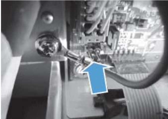
Figure 3-98 Ground wire for ADF cable
