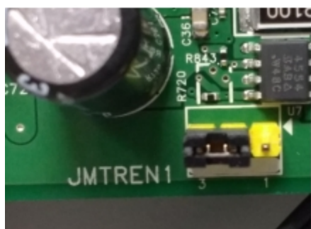
Interlock bypass disabled (default)
