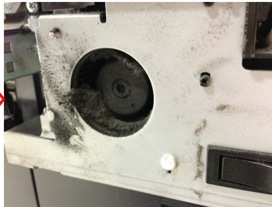
Before (With clogging)
