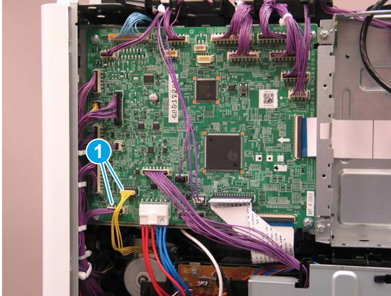
Figure 1-1313 Check the yellow cable
